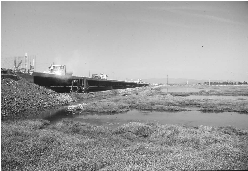
Fig. 1: The viaduct under construction (2002), seen from the 'Orti' brackish marsh. Piombino, Province of Livorno, Tuscany, Italy.
